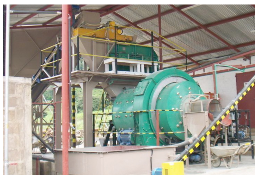
The 2.5t/hr ball mill operating at only 34% capacity on site
