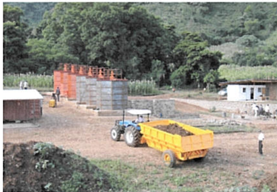
Tailings retreatment tanks, agitators and necessary retreatment equipment are in production.
