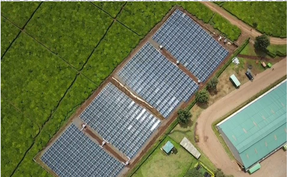
A 1 MW plant in Nandi Tea Factory, installed by Equator Energy
